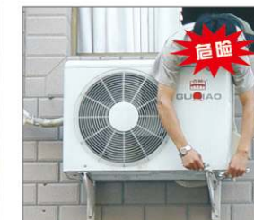
Very dangerous 非常危险
